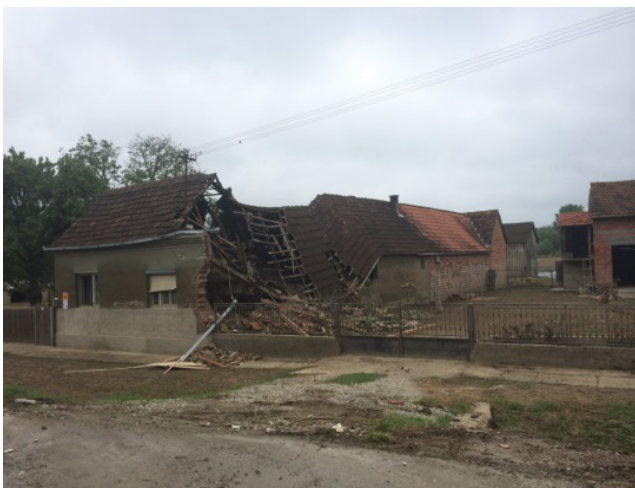
Figure 6: The damage magnitude in village Račinovci.
