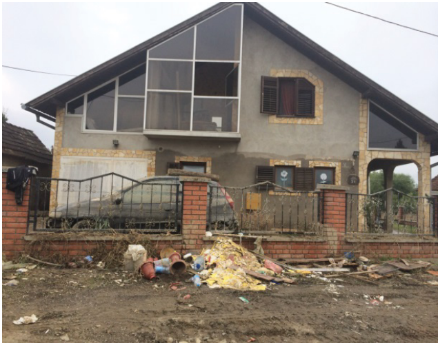
Figure 4: Flood affected house in village Gunja.
