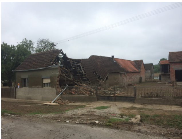
Figure 6: The damage magnitude in village Račinovci.
